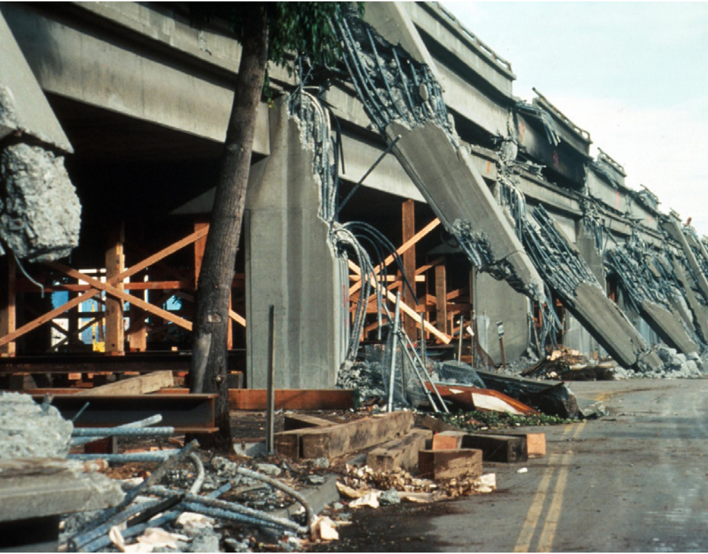
Figure 3. Support column failure and collapsed upper deck on the Cypress viaduct of Interstate 880 caused by the October 17, 1989, Loma Prieta earthquake. Photo by H. G. Wilshire, USGS.
