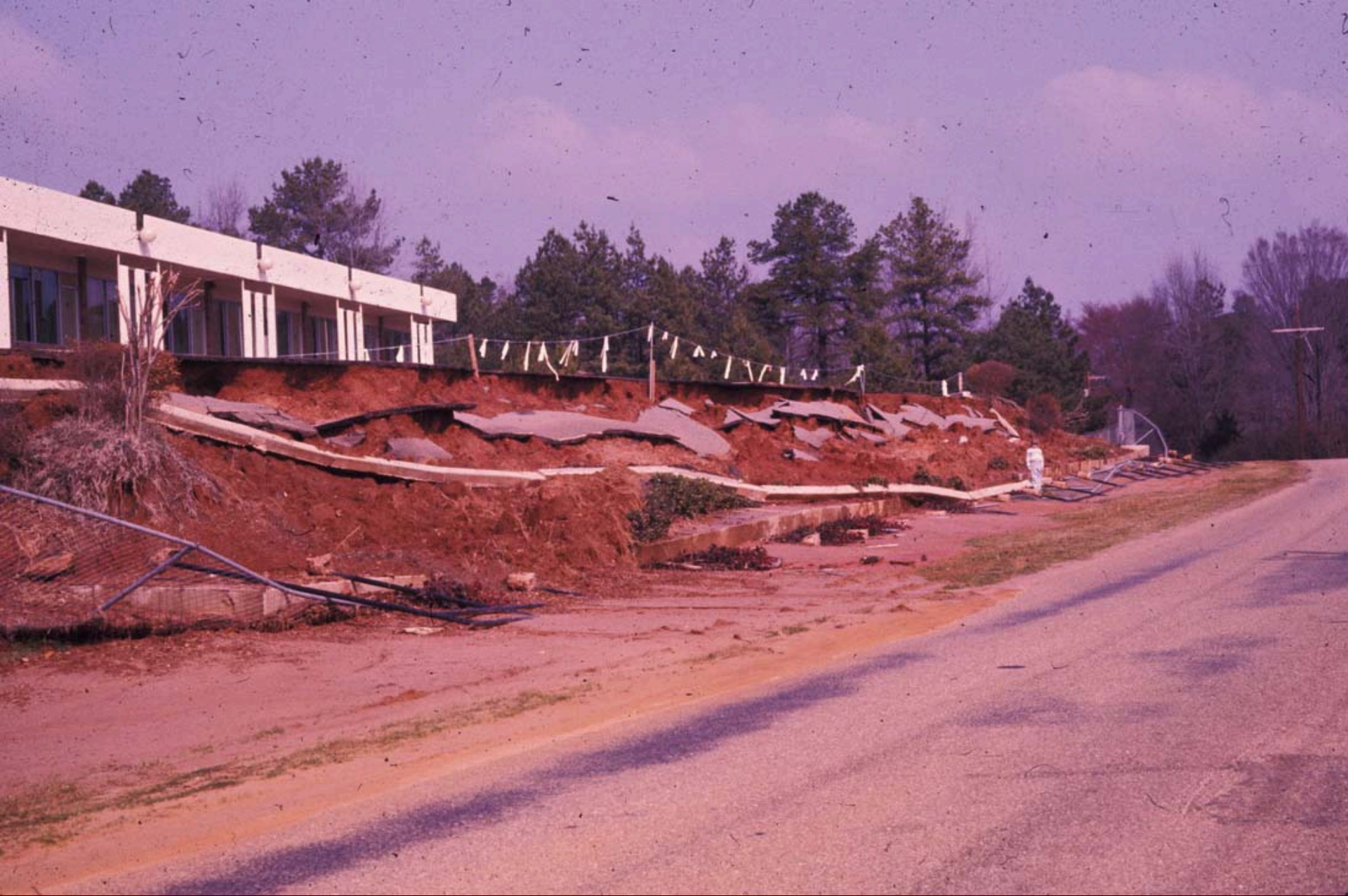
Wall failure at Holiday Inn, Ruston after 12 inches of rain in two days
