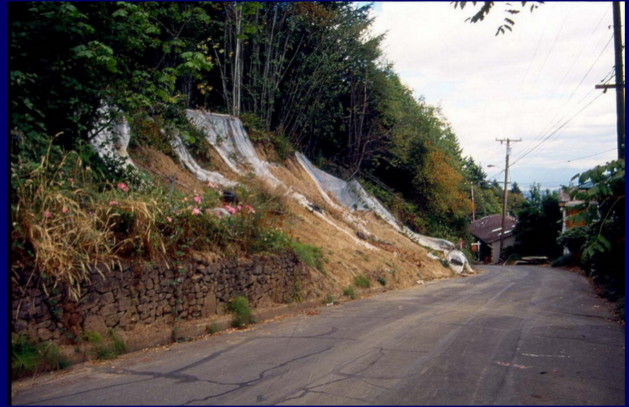
Street Drains Clogged: World’s Fastest Earthflow at Pittock Mansion
