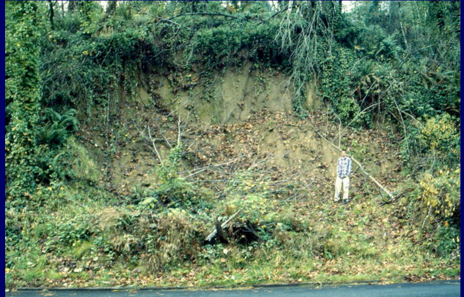
Landslide before fix
